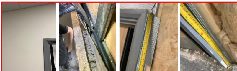
Cracking example and investigation works
